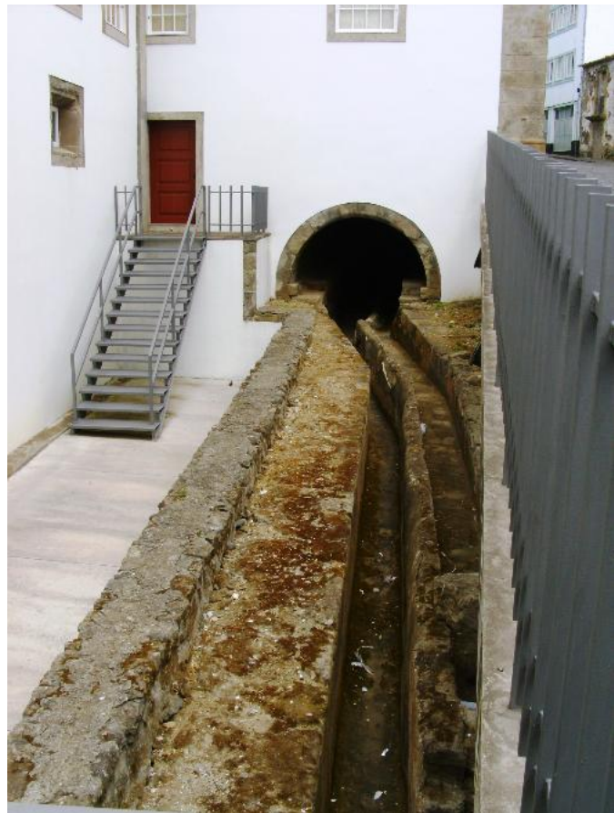
In the old Monastery of S. Francisco (the Museum) two pipes can still be seen: one to provide fresh water, the other to be used as sewage.
